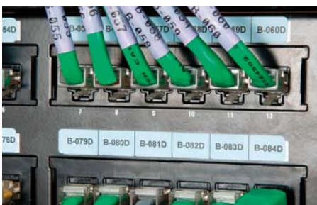
Patch Panel Labels
