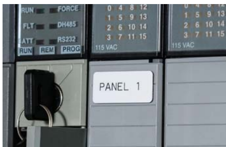
Control Panel Labels
